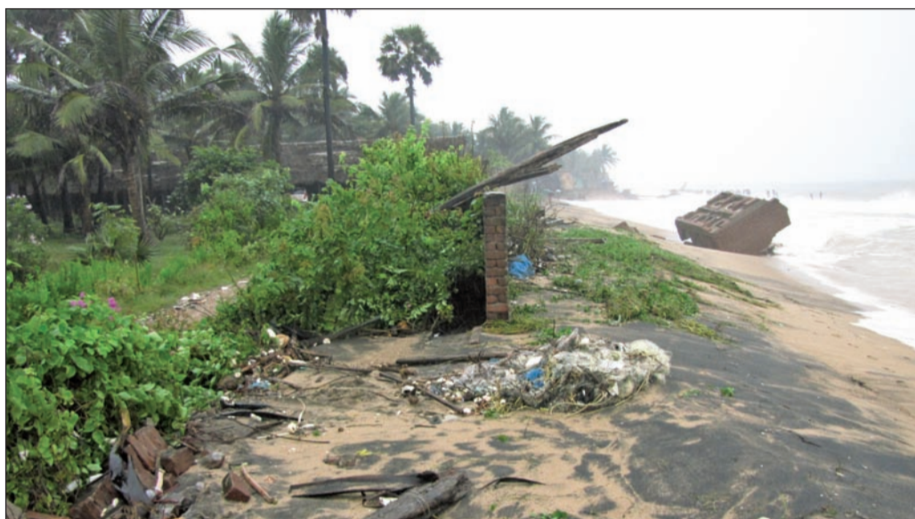
The beach in front of Quiet in November 2010. The compound wall has crumbled.
