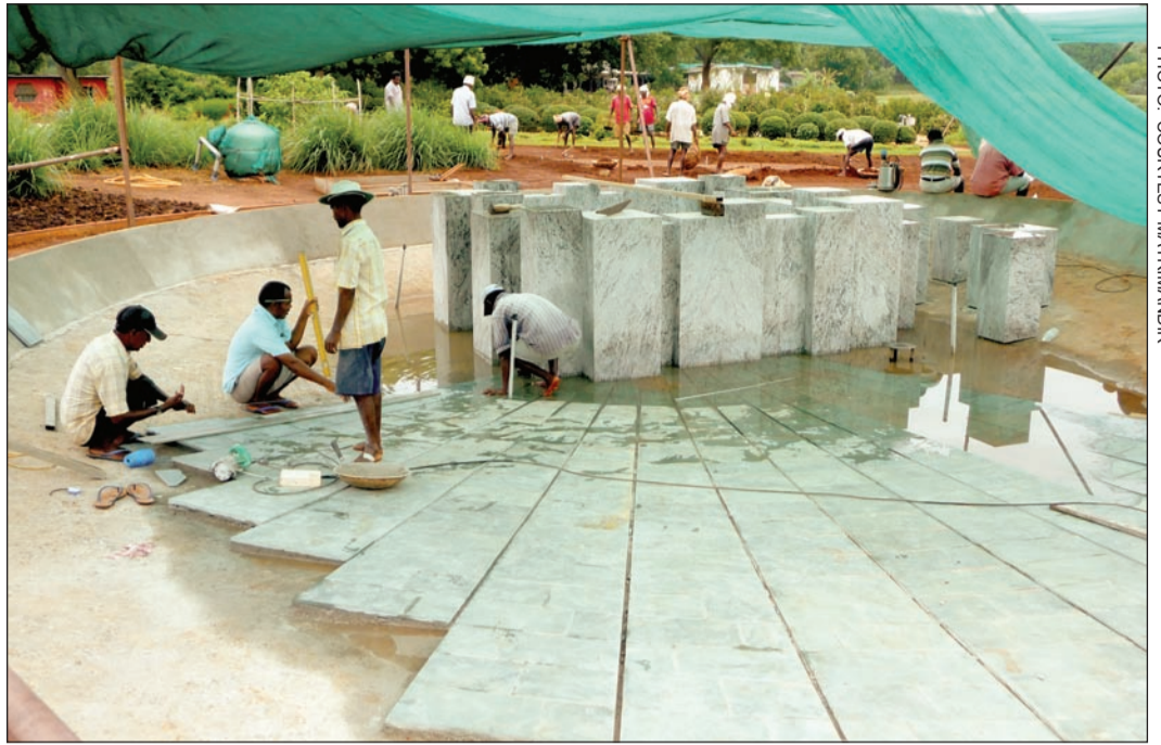
PHOTO: COURTESY MATRIMANDIR Work on the pool in the Garden of Consciousness is almost completed
