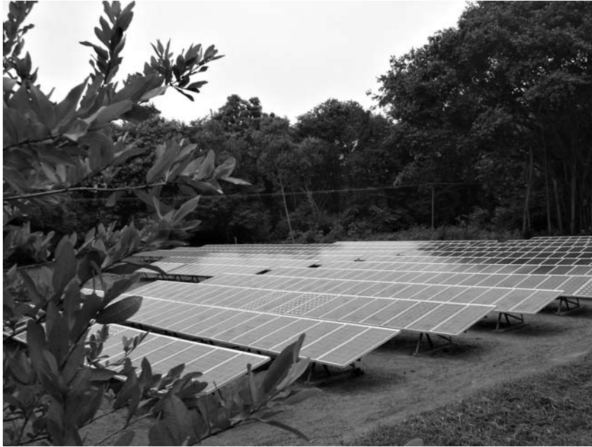
Panels of the solar power plant located outside the Oval
